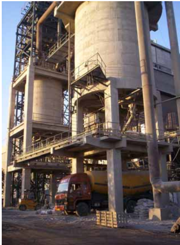
Dry Fly Ash Collection And Classification Unit At Dahanu Thermal Power Plant
